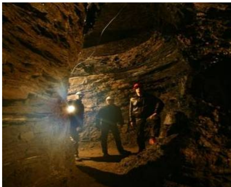
Photo 71: “KTK” underground tunnel after cleaning; total of 150 meters were cleaned and secured. Main tunnel is located between two rivers (river Bosna and river Fojnica) and goes in direction of the Bosnian Pyramid of the Sun
